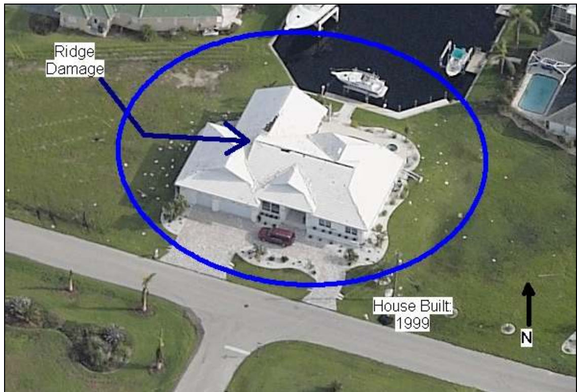
Figure A.4: Wind Damage Done to Ridges (Property #4)
