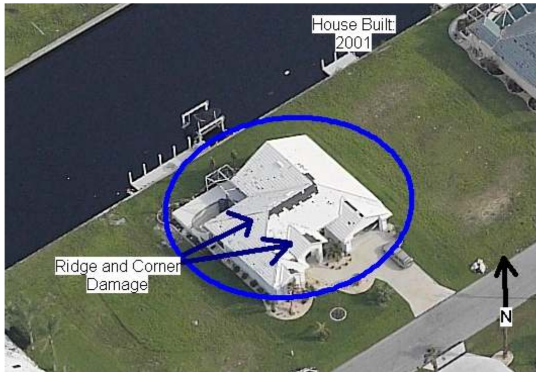
Figure A.7: Ridge and Corner Damage (Property #7)
