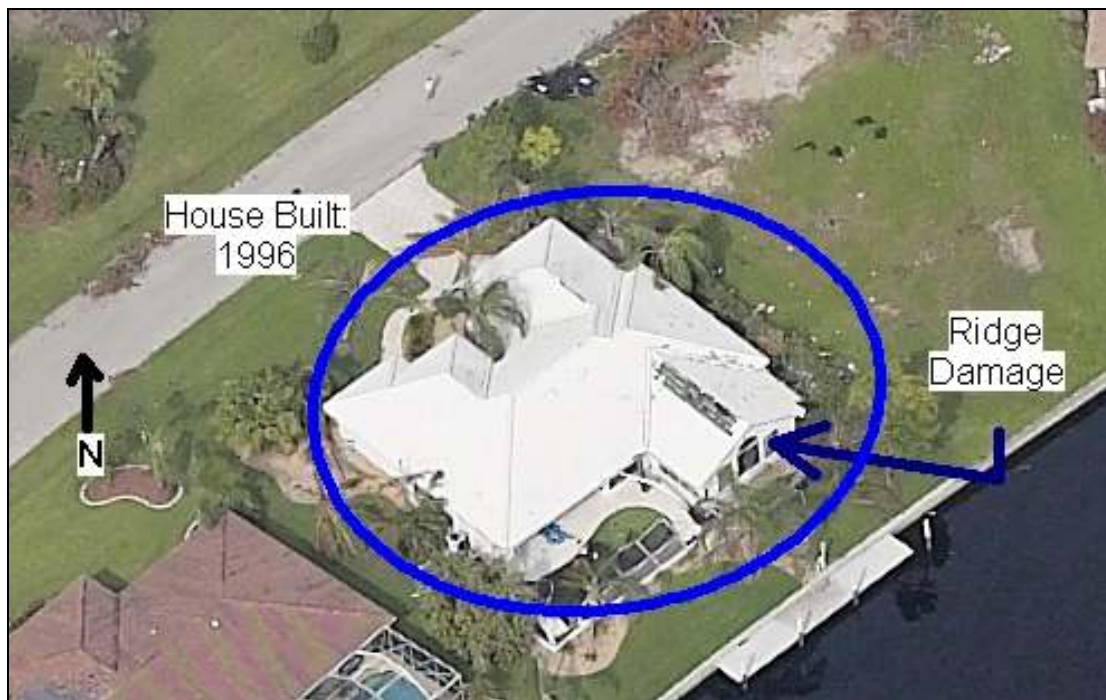
Figure A.2: Wind Damage Done to Ridges (Property #2)
