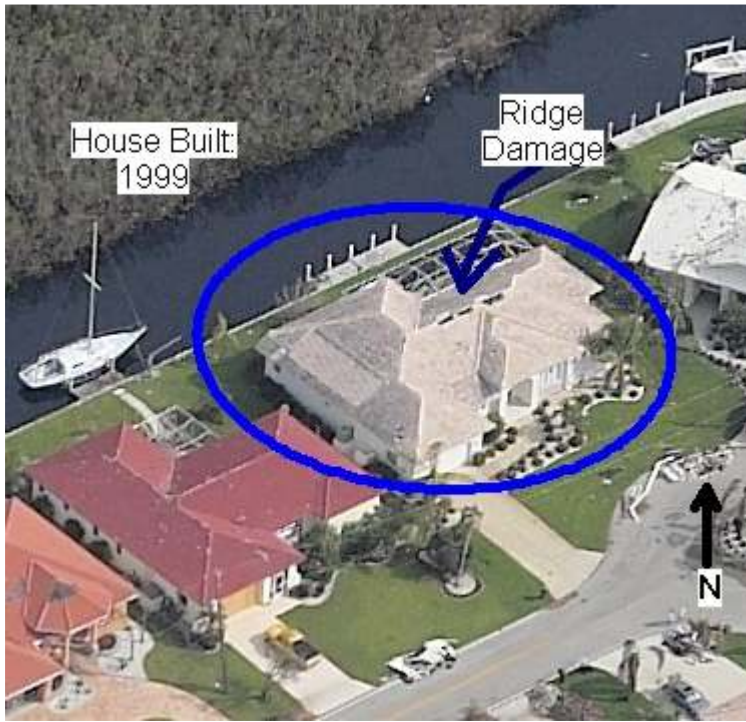
Figure A.19: Ridge Damage (Property #19)
