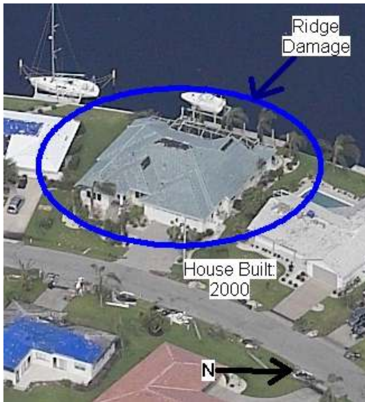
Figure A.9: Ridge Damage (Property #9)
