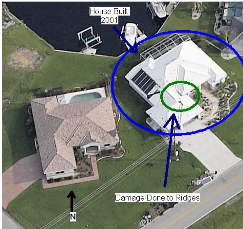
Figure A.11: Ridge Damage (Property #11)
